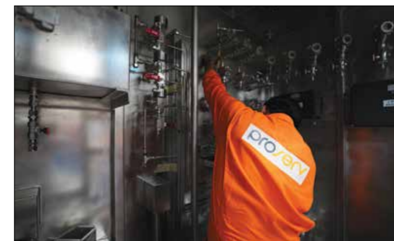
A Proserv technician inspects core equipment
